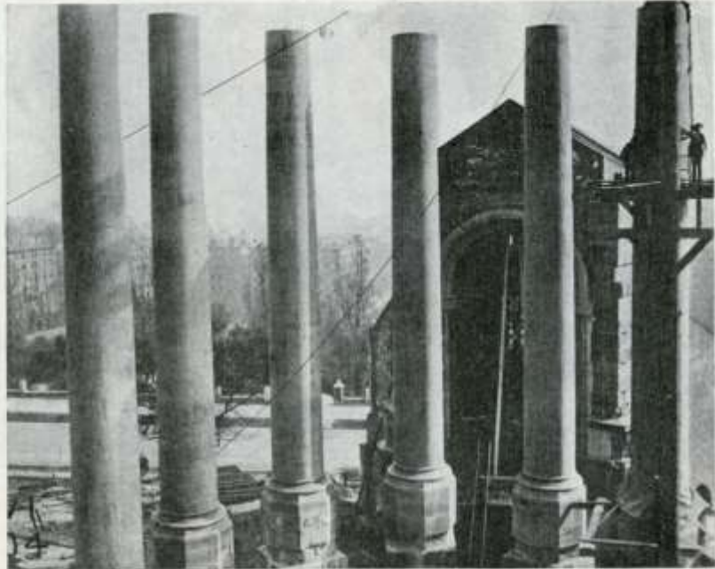
SETTING THE SIXTH COLUMN IN CATHEDRAL OF ST. JOHN. The Columns are Inside the Church; Arranged in a Semi-Circle.
