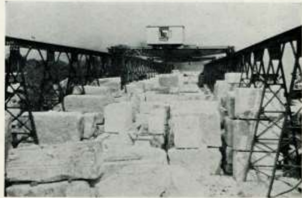
Stock Yard and Crane-way of F. W. Steadley & Co., Inc., 1,000 feet long and equipped with two thirty ton cranes.
